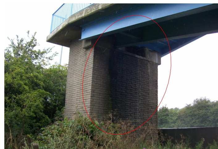
Photograph 2 Staining due to water leakage
