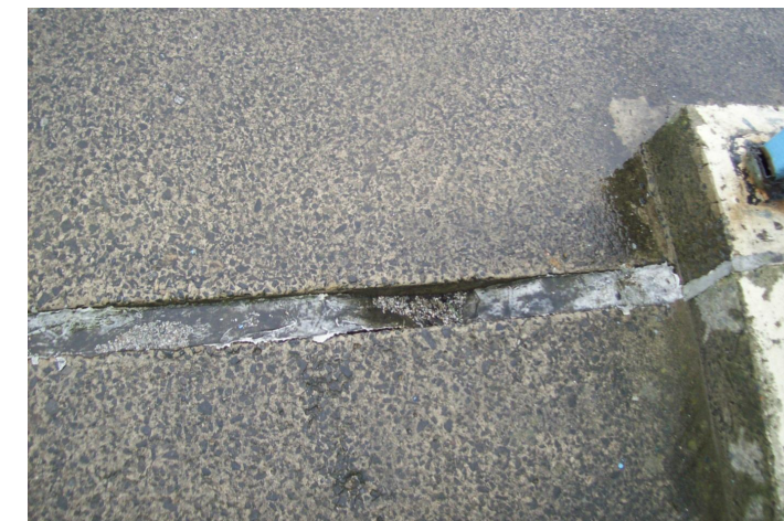
Photograph 3 Deterioration of bridge joint
